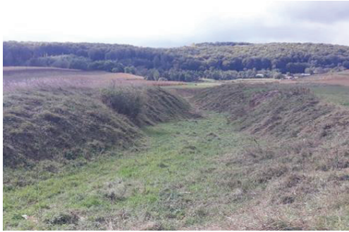
Figure 7. A stabilized gully erosion on arable land in Forăști
