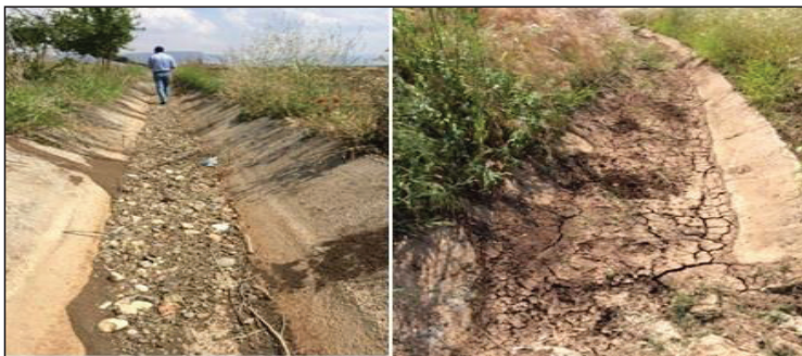
Figure 10. Problems of gravel and soil residues that accumulate in irrigation channels
